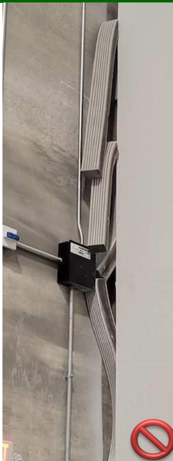
The Silicone/foam joint was installed incorrectly and most likely the wrong size to accommodate the movement of the panels.
