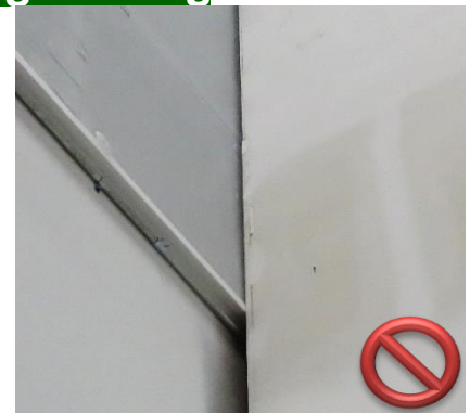
Electrical conduits and insulation panels cannot be within the fire rated joint. The insulation needs to be cut before and after the interior partition.
